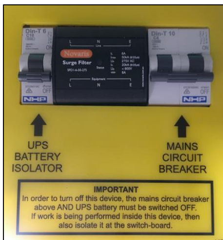
Figure 2: TT8800 OPT Breaker Panel
